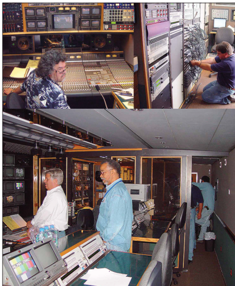
Figure 3.28 A walk through a "show" truck. The top two pictures are the audio compartment and the equipment and transmission areas, which are at opposite ends of the trailer. The audio compartment is large enough to accommodate not only the A1 shown here, but also a couple of A2s to handle sub-mix duties on a large music show. The bottom picture shows part of the production compartment in the foreground, with tape (left) and video (right) toward the rear.
